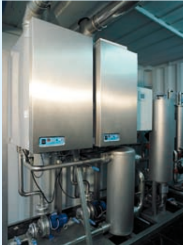
Aquaheater with a capacity of 2x180 kW
